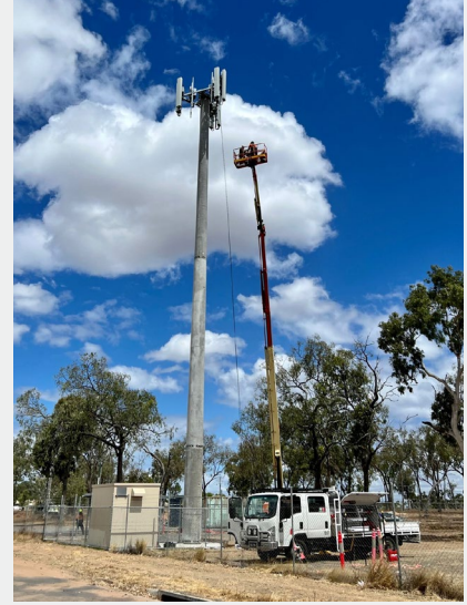
New mobile data infrastructure is being built in Dysart and Moranbah through the Digital Connectivity Project.
