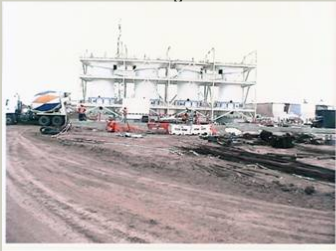
Ultra-fines microcell tanks
